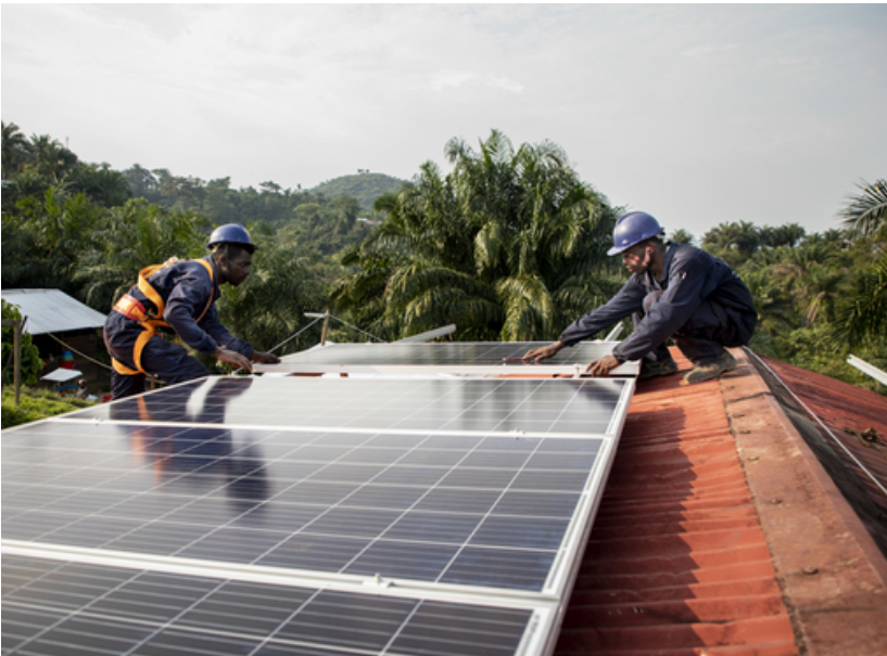
© Pablo Garrigos for MSF. MSF has settled a solar panel system at the General Hospital of Kigulube in Sud Kivu, DRC to give autonomy to the health structure for the next 20 years.
