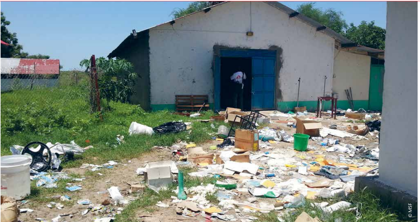
The MSF hospital in Pibor after it had been purposefully damaged to render it inoperable.
